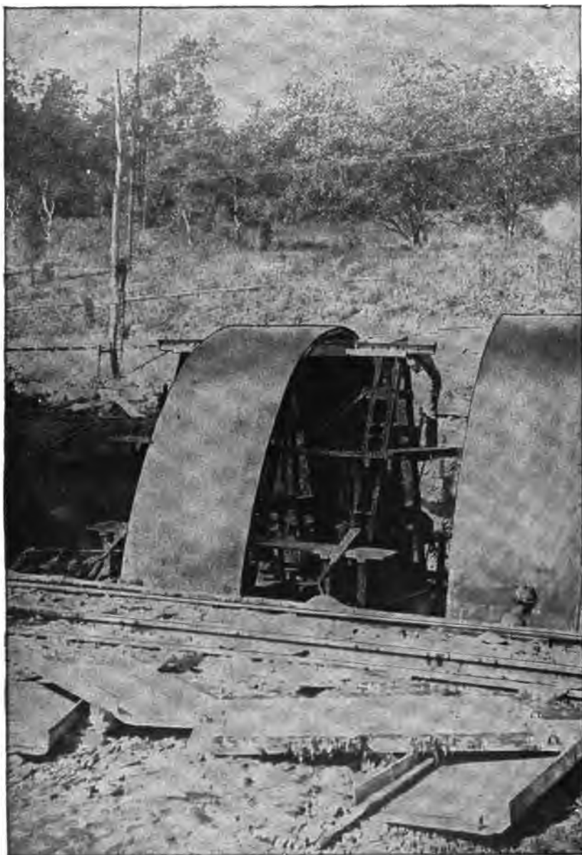
PLATE 127.—Section of Inside Form—5 Feet—Being Moved to New Position and Turned around to Form Curve. Sections are wedge-shaped for 200-foot radius curve.
